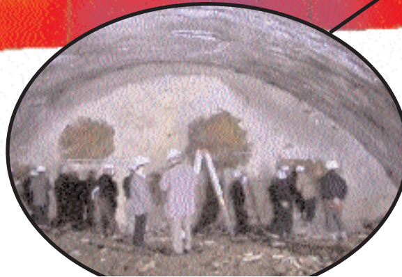
The tunnel front at the weak zone was shot-creted and three windows left open for the engineers to study the weak-zone material.
